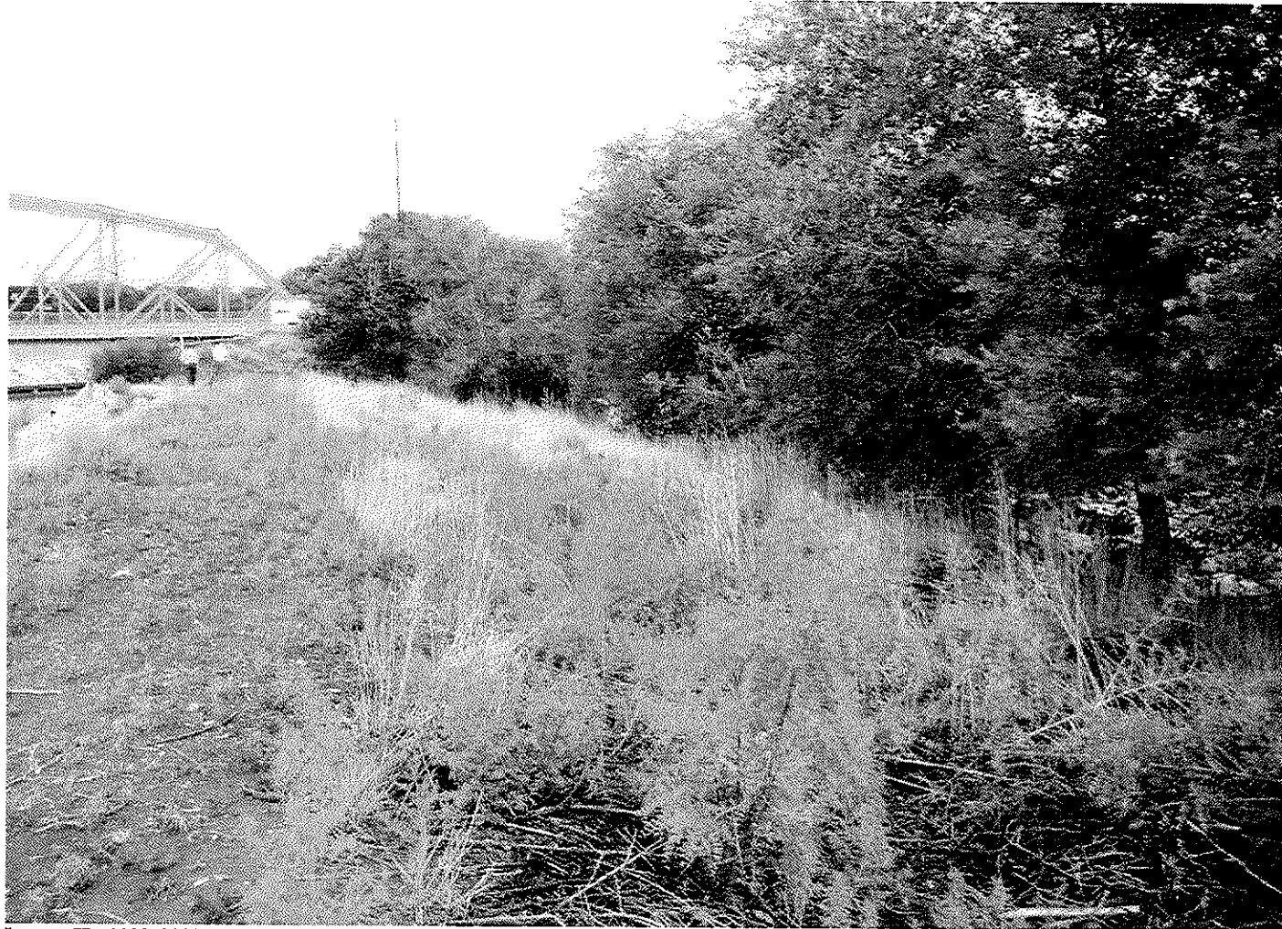
Inspect ID: 0008_2008_a_0006 Name: USACE_CESPA_0008_2008_a_0006_3.jpg Caption: Trees growing along levee.
