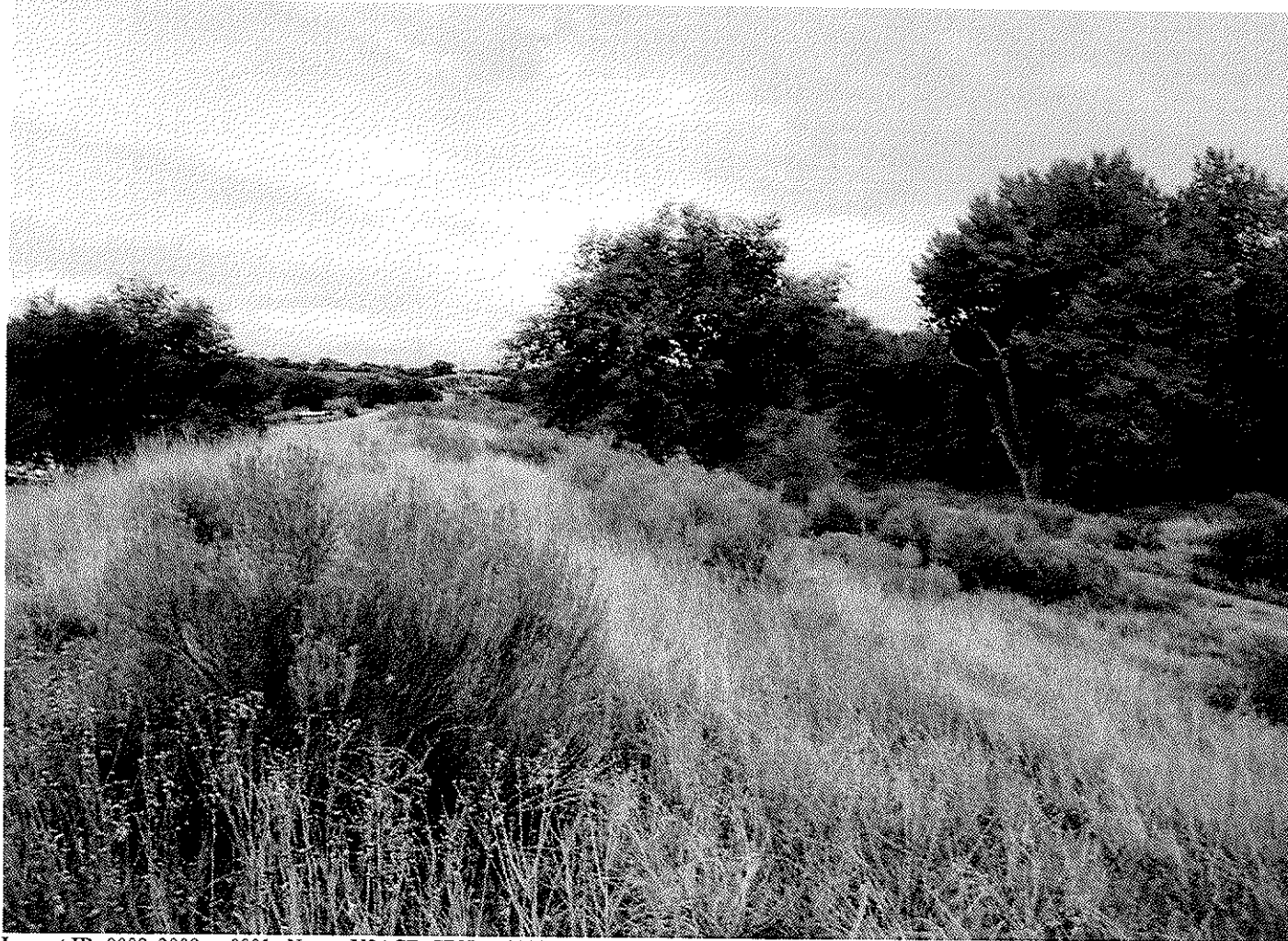
Inspect ID: 0008_2008_a_0001 Name: USACE_CESPA_0008_2008_a_0001_1.jpg Caption: Bushes on levee crest and trees at toe.
