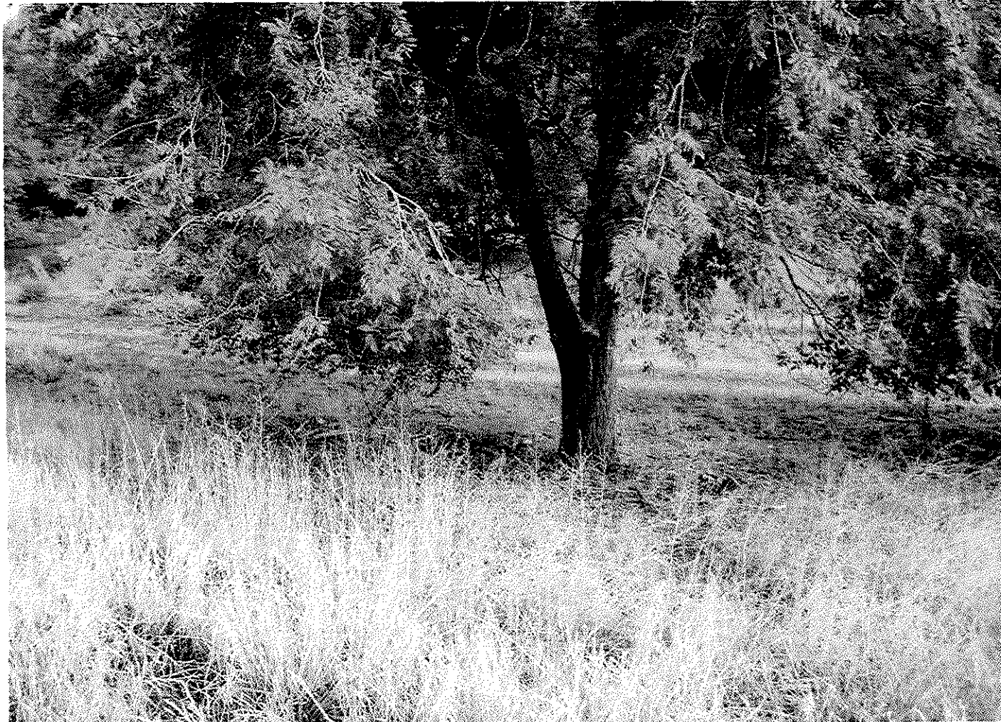
Inspect ID: 0008_2008_a_0001 Name: USACE_CESPA_0008_2008_a_0001_2.jpg Caption: Tree at levee toe.
