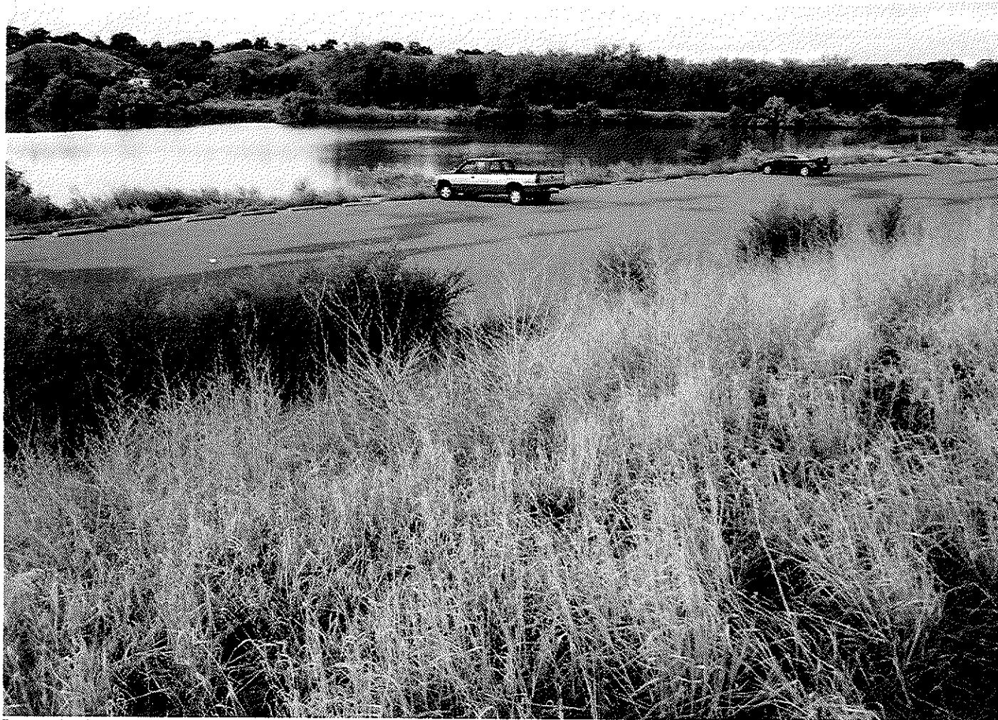
Inspect ID: 0008_2008_a_0003 Name: USACE_CESPA_0008_2008_a_0003_1.jpg Caption: Trees growing at levee toe.
